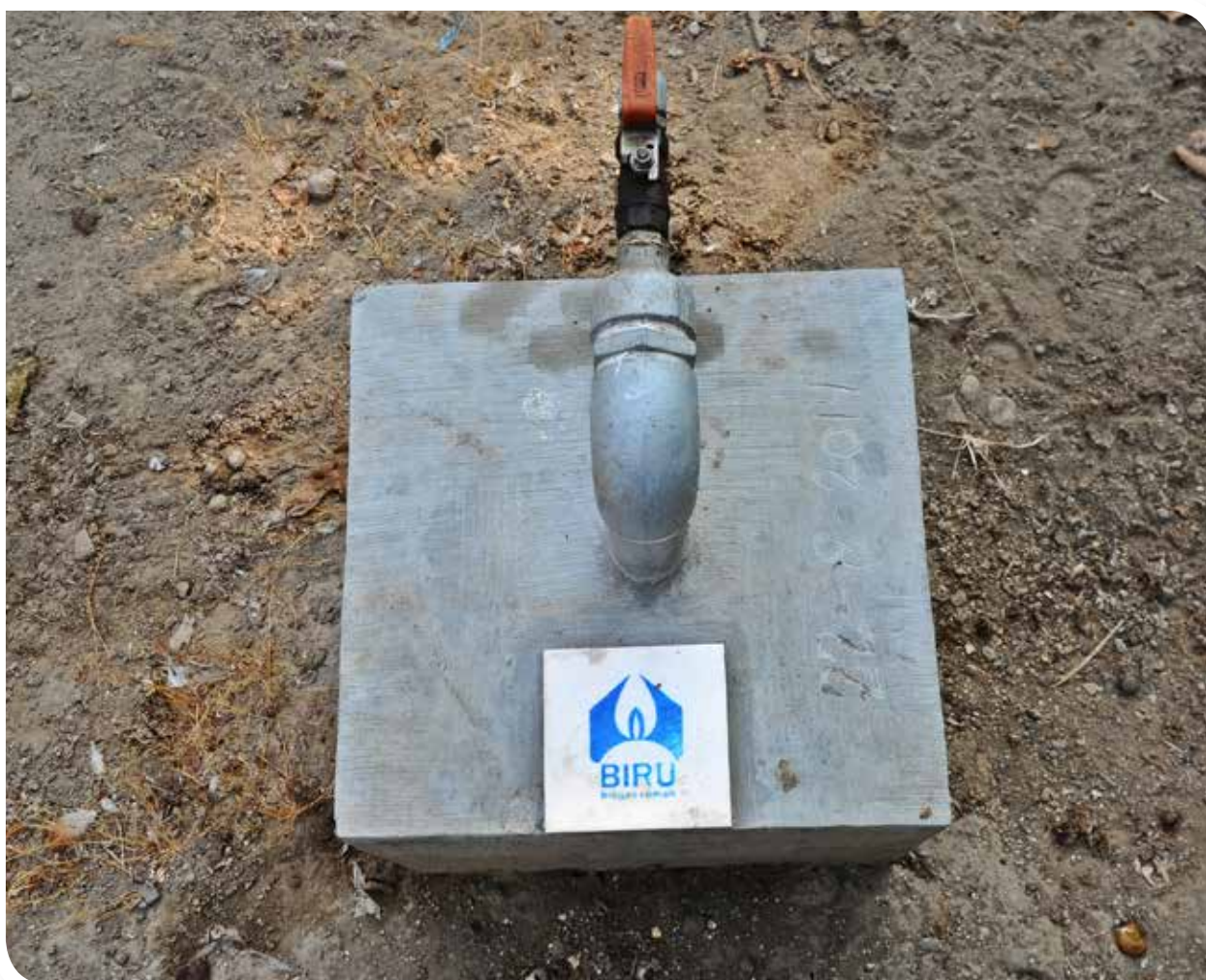
IDBP installation in Kediri, East Java (photo by Rumah Energi)
